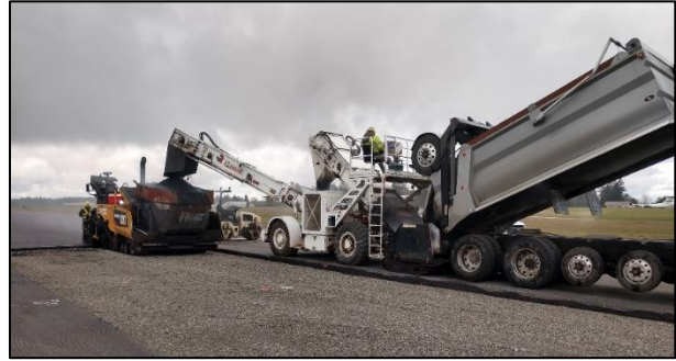
Figure 8: Material Transfer Vehicle in Use during Runway Paving at Joint Base Lewis-McChord, Washington. Photo courtesy of the USAF.
