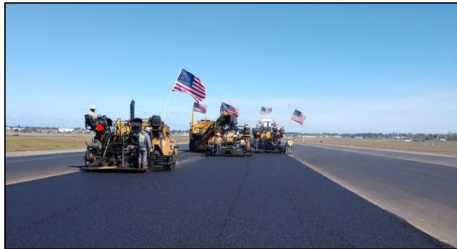
Figure 7: Echelon Paving on Joint Base Lewis-McChord, Washington. Photo courtesy of the USAF.
